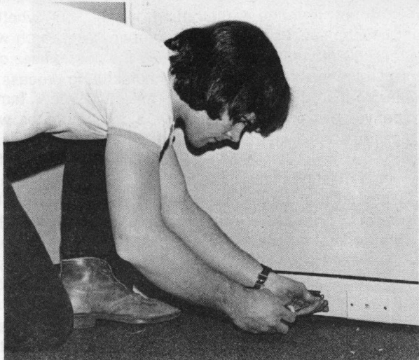
Electrician's Helper Kerry Moore encloses all wiring in base of modular office.
